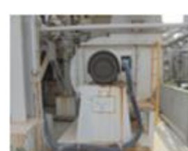
Exhaust fan runner (after)
