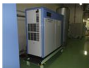
Compressor(after) Case 4 (Nagasaki Facility)
