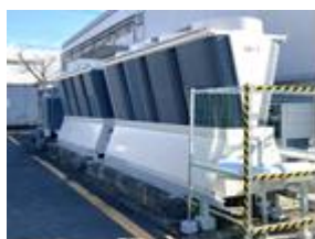
Chiller (after) Case 2 (Hadano Facility)
