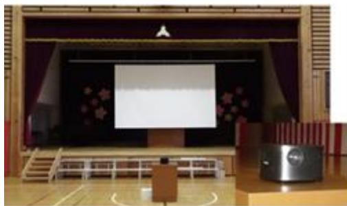
Photo of the projector installed in the gymnasium of Oguni Elementary School (Oguni Facility)
