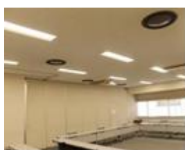
LED lamp(after) Case 1 (Oguni Facility)
