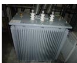
transformer(after) Case 1 (Oguni Facility)
