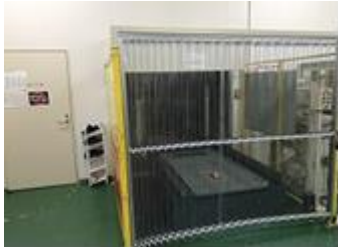
A guarding with an interlock is installed at the doorway of the auto stocker. (Oguni Facility)
