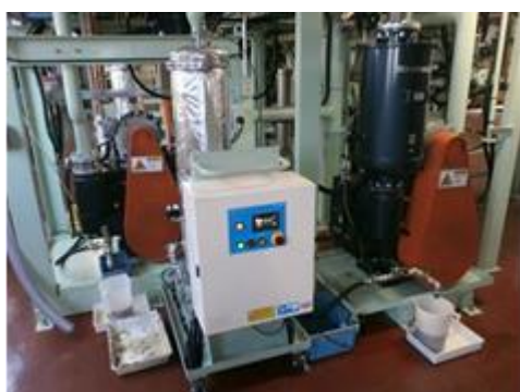
Filtering equipment (Kariya Facility)
