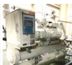
Chiller (after) Case 3 (CoorsTek Tokuyama)
