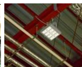
LED lamp(after) Case 4 (CoorsTek Nagasaki)
