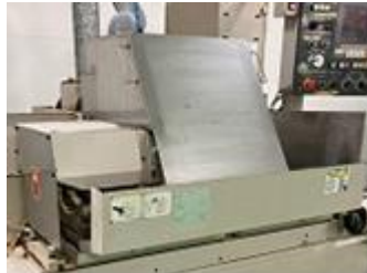
Minimize the exposure of the rotating parts of the processing machine, and install a guarding on the outside of the device. (Kariya Facility)
