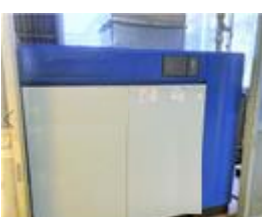
compressor(after) Case 2 (Kariya Facility)
