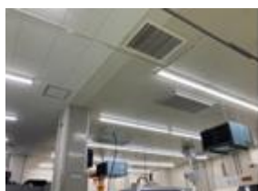
LED lamp(after) Case 2 (Hadano Facility)
