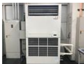
Air conditioner(after) Case 1 (Oguni Facility)
