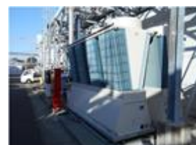
Chiller (after) Case 5 (CoorsTek Nagasaki)
