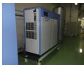
Compressor(after) Case 4 (Nagasaki Facility)
